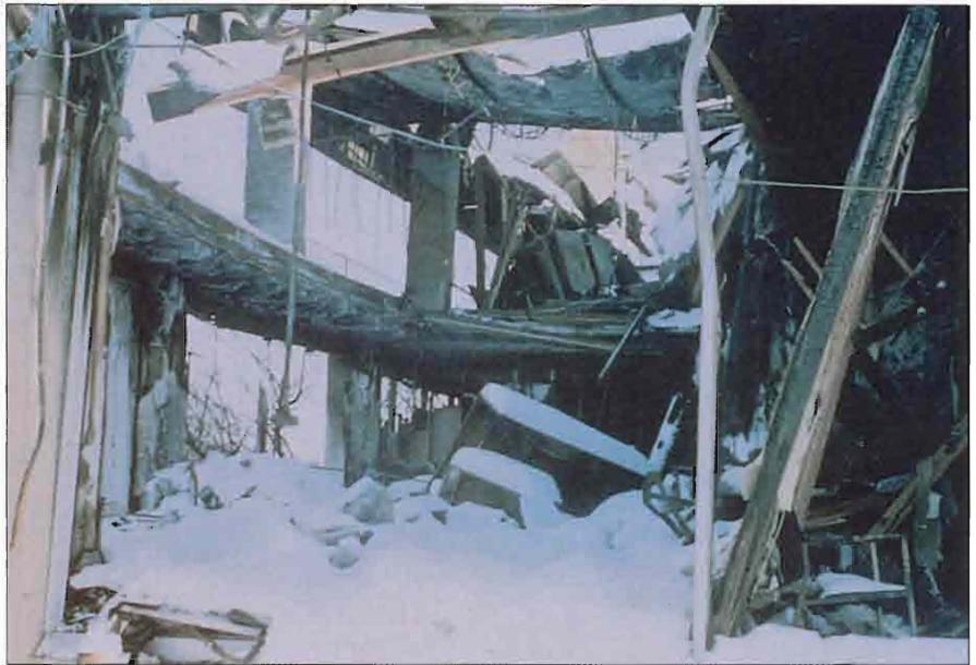
This computer facility collapsed under heavy snow.
